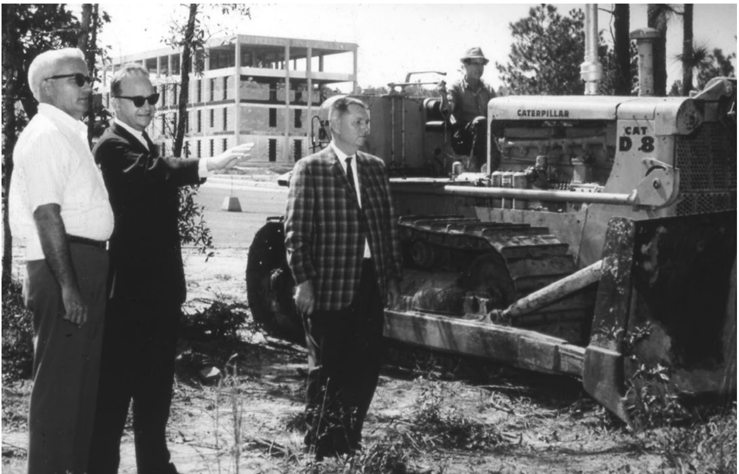
Dr. Fred Whiddon, center, and Dr. James Caldwell, vice president for development, at right, look over construction for a new building. Photo courtesy of The Doy Leale McCall Rare Book and Manuscript Library.
